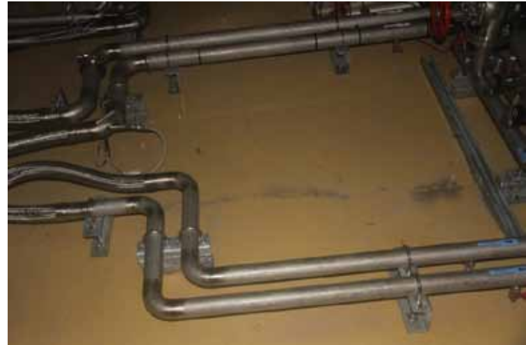
Crack observed on March 28 after pumping water.
