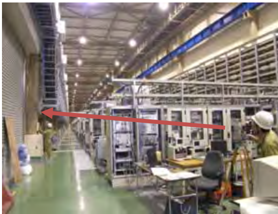
Measurement by laser for Klystron (10 mrad distortion toward west side was observed) .
