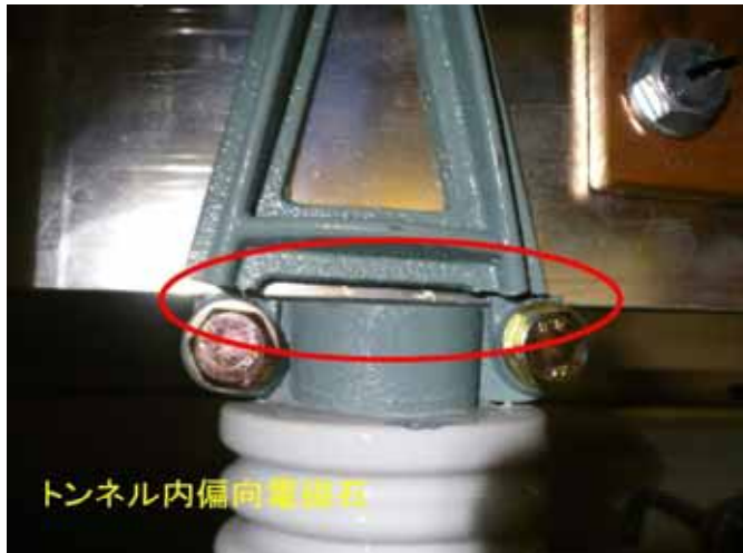
Casting that was broken (Dipole magnet)
