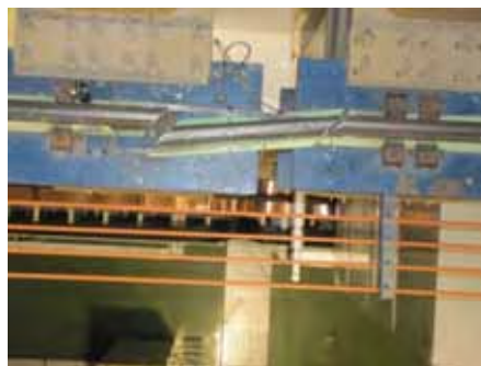
Crane rail in the Klystron Gallery (partial damage detected).
