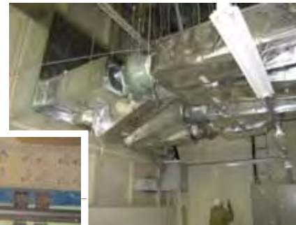
Air conditioning Pipe is falling down.
