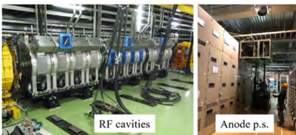
Fig. 16. Upgrade of the RF systems.
