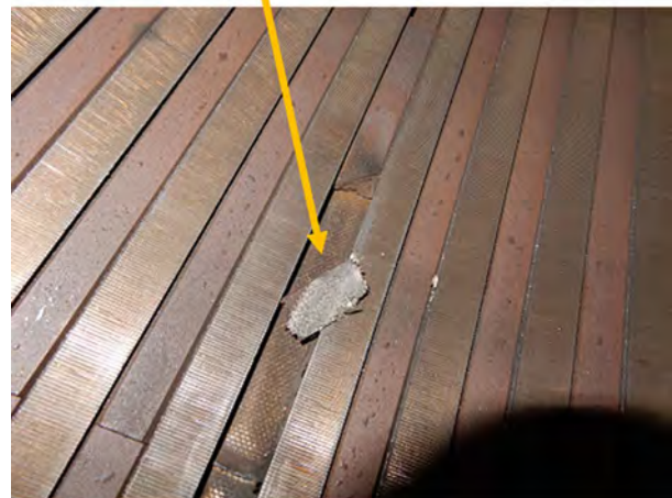
Fig. 12. Inside of the broken pump. A coil support was broken.
