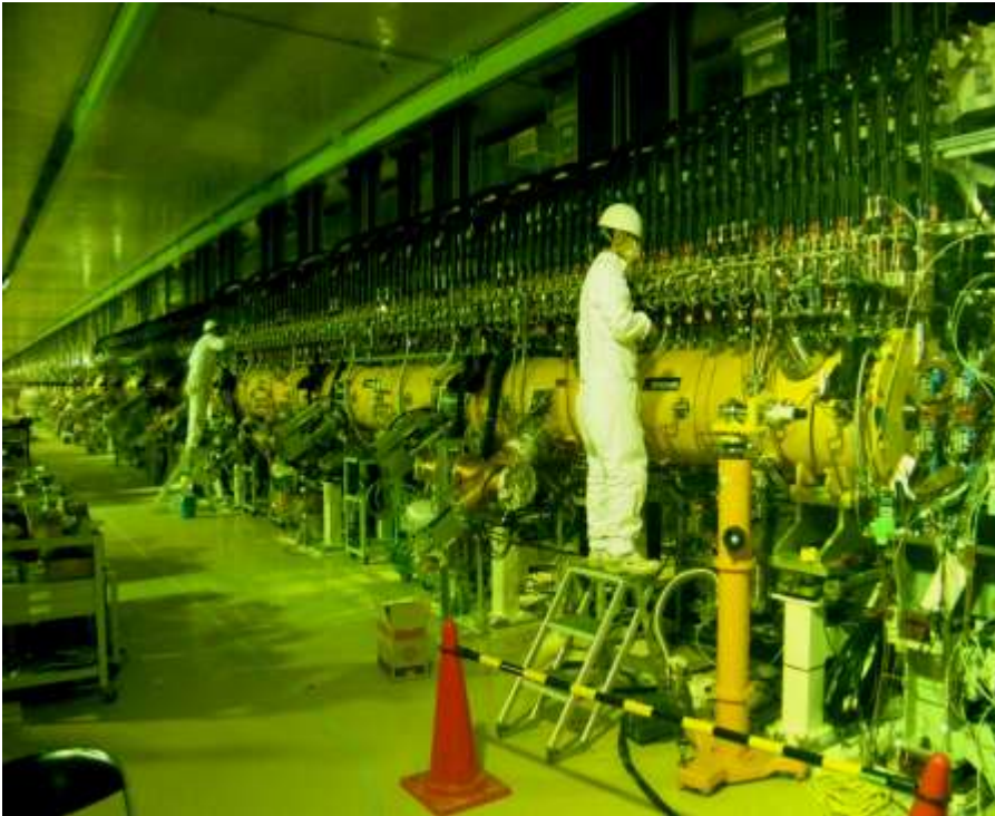
Realigned accelerator cavities of DTL and SDTL were tested for water-tightness.
