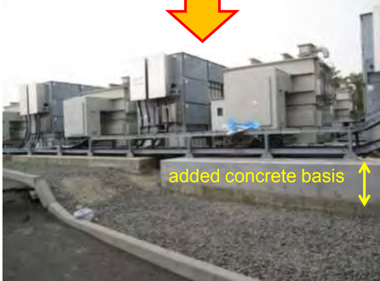
Tilted condensers were straightened after relabeling the bases.
