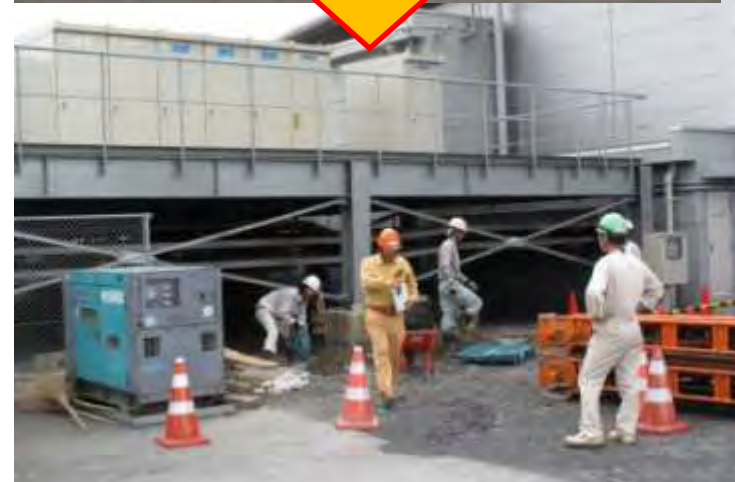
The bent stage was repaired. Power has been supplied to the RCS building.
