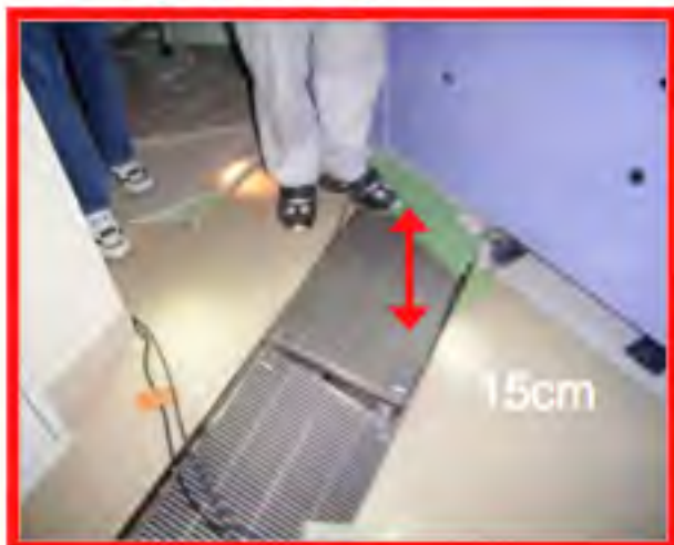
Sinkage of building
